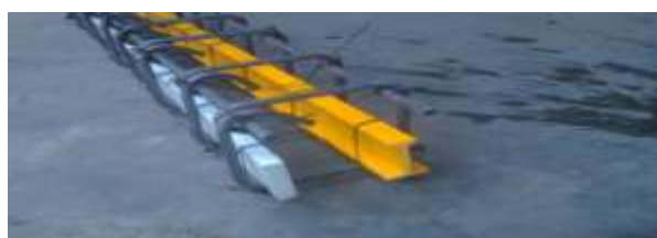
Fig 9.5 Reinforcement details for beam reinforced with combination of GFRP plate and I-section (GPI)
